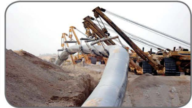
IGAT V – Gas Trunk line
