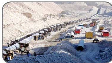
IGAT V – Gas Trunk line
