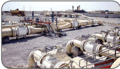
Station No.5 Gureh- jask Pipeline
