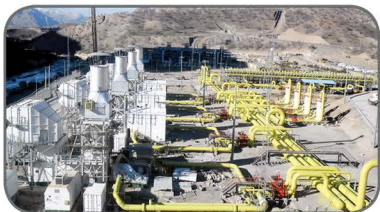
Pataveh 4 Gas Compressor Station
